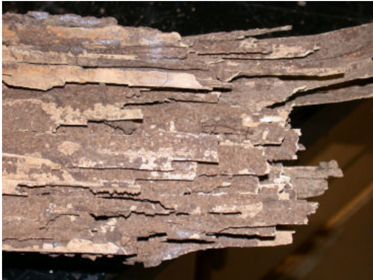
Damage to wooden beam--note mud caked on wood.
